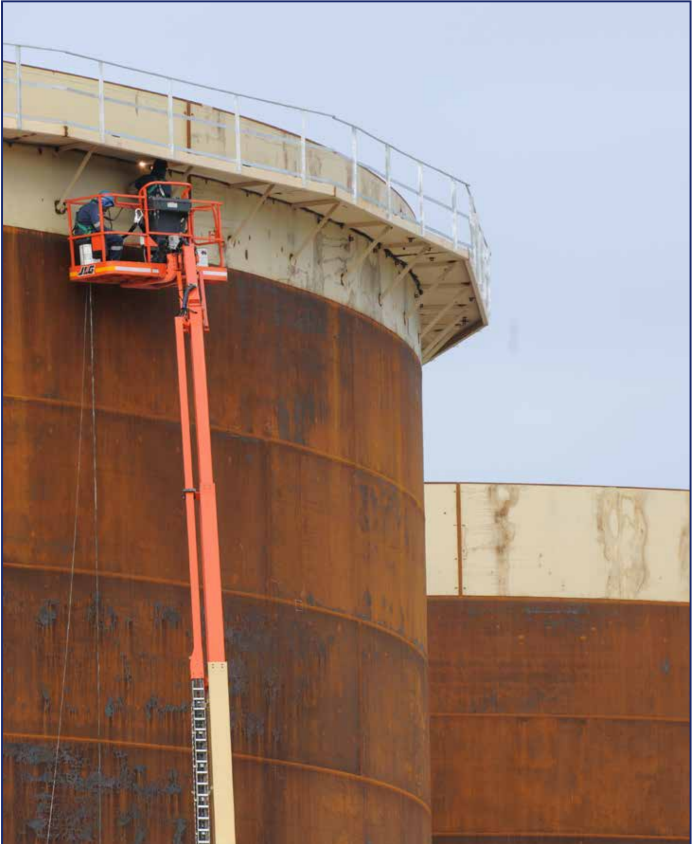
Orion Engineered Carbons Black Oil Tank Project in Zone 7 of the Coega SEZ.
