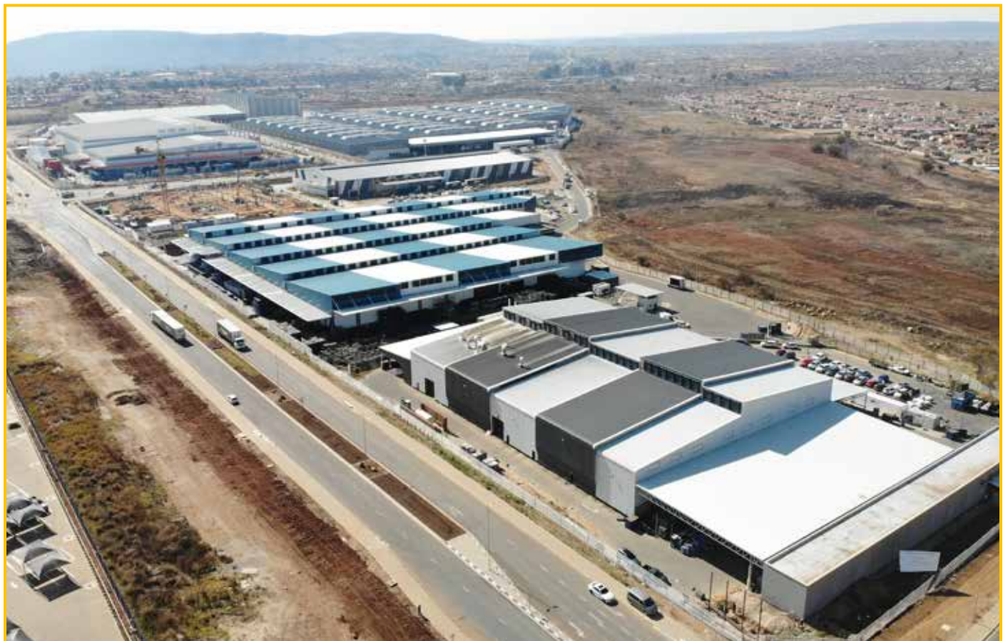
Tshwane Automotive Special Economic Zone construction update, with Coega as the Infrastructure Implementing Agent of Choice: A Case Study for South Africa's Infrastructure Development Excellence.
