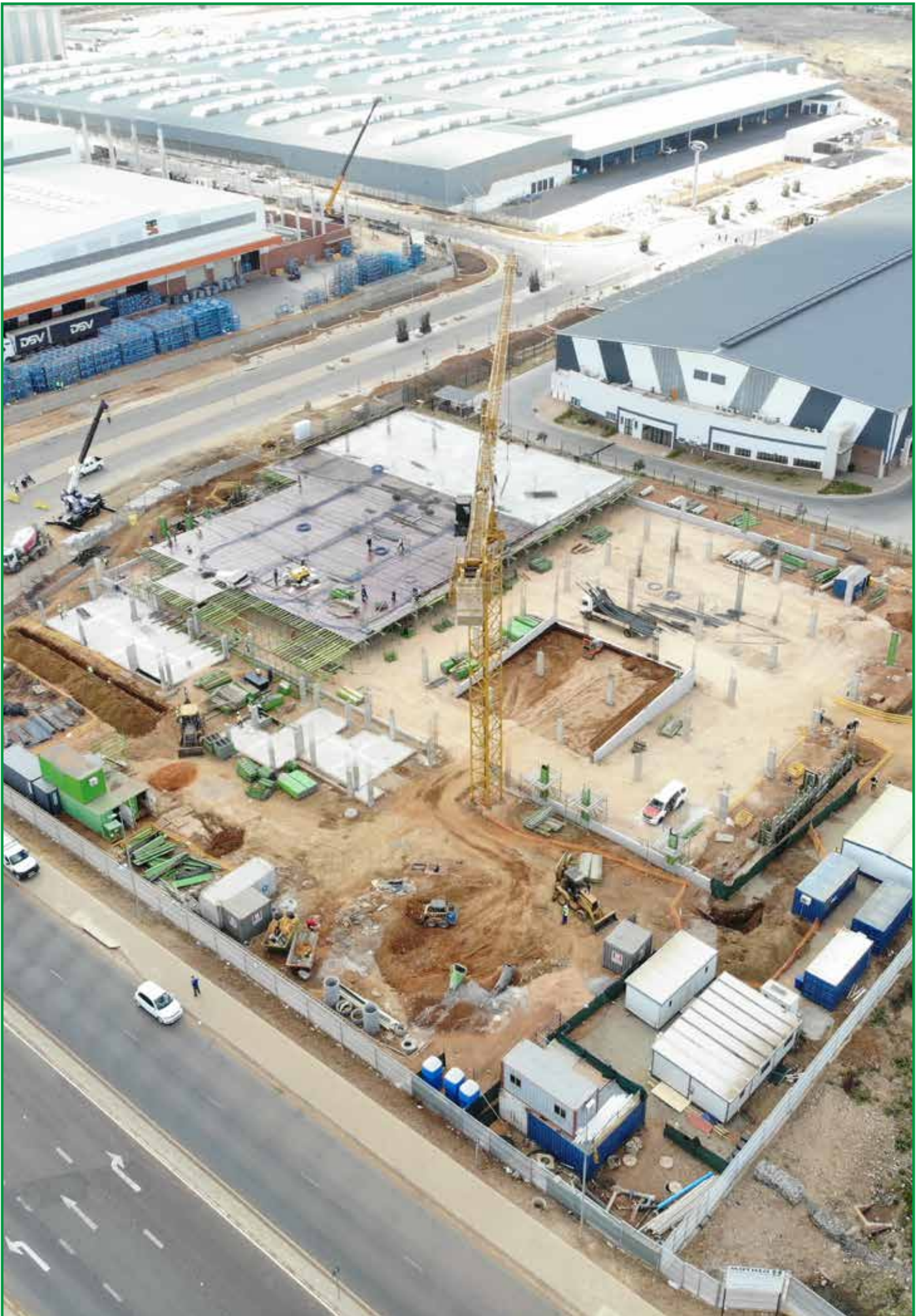
Tshwane Automotive SEZ Central Hub construction site, with Coega as a trusted infrastructure implementing agent of choice, in partnership with Gauteng Provincial Government, the dtic, and City of Tshwane. Visit www.tasez.co.za .
